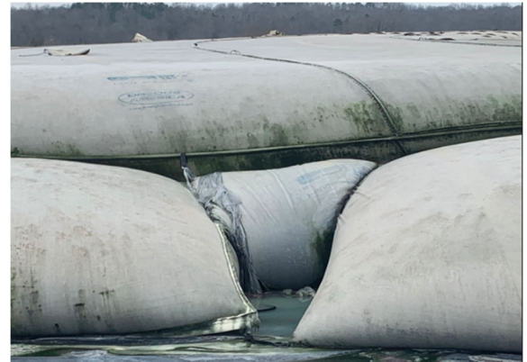
Example of a stacked application with filler tubes used to fill void space in base layer
